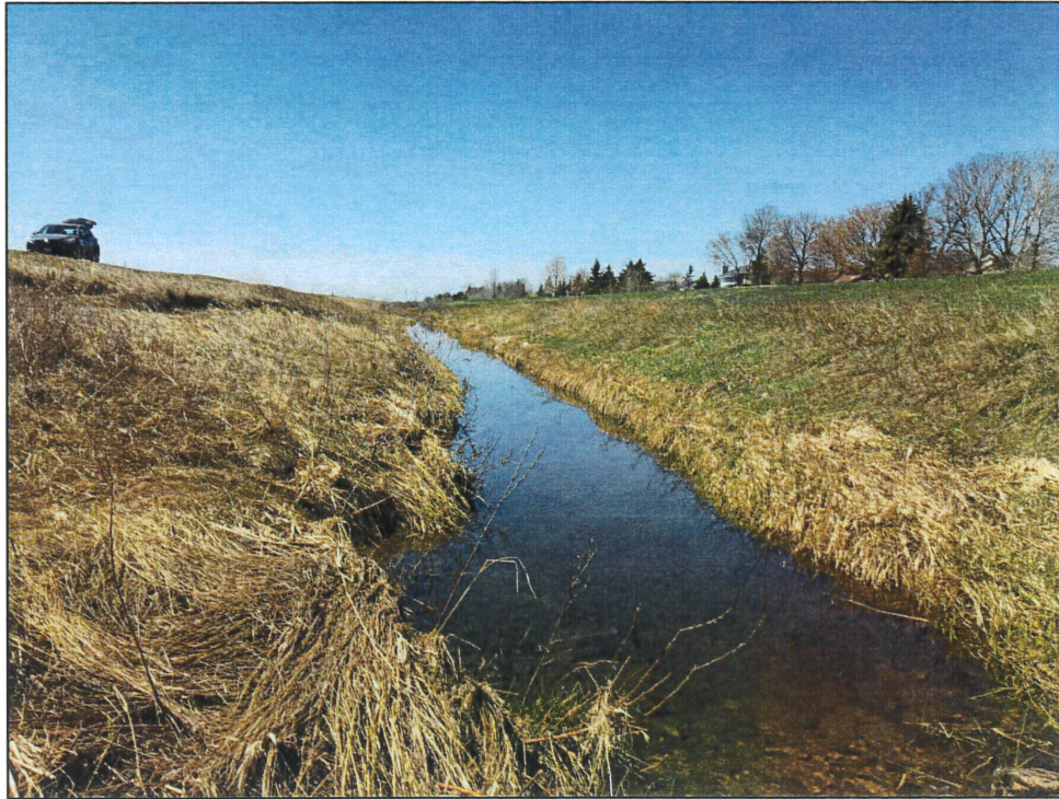
PHOTOGRAPH 3: FACING SOUTH WEST SHOWING ONE OF THE AREAS OF THE BANK WITH SEVERE FAILURE
