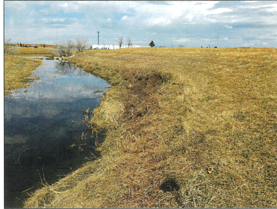
PHOTOGRAPH 4: FACING NORTH EAST SHOWING ONE OF THE AREAS OF THE BANK WITH SEVERE FAILURE
